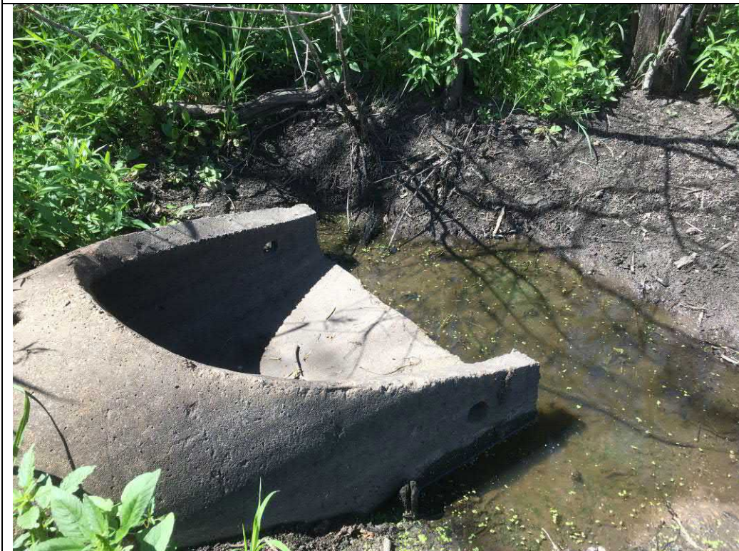
CUSICK PARKWAY CULVERT PERCHED ABOVE STANDING WATER (NO FLOW).
