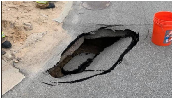
Sinkhole in need of repair
