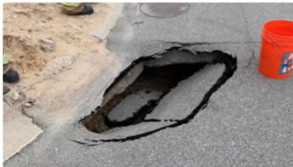
Sinkhole in need of repair
