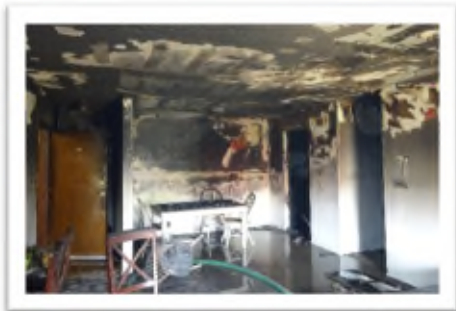
High Ridge Trail Kitchen Fire
